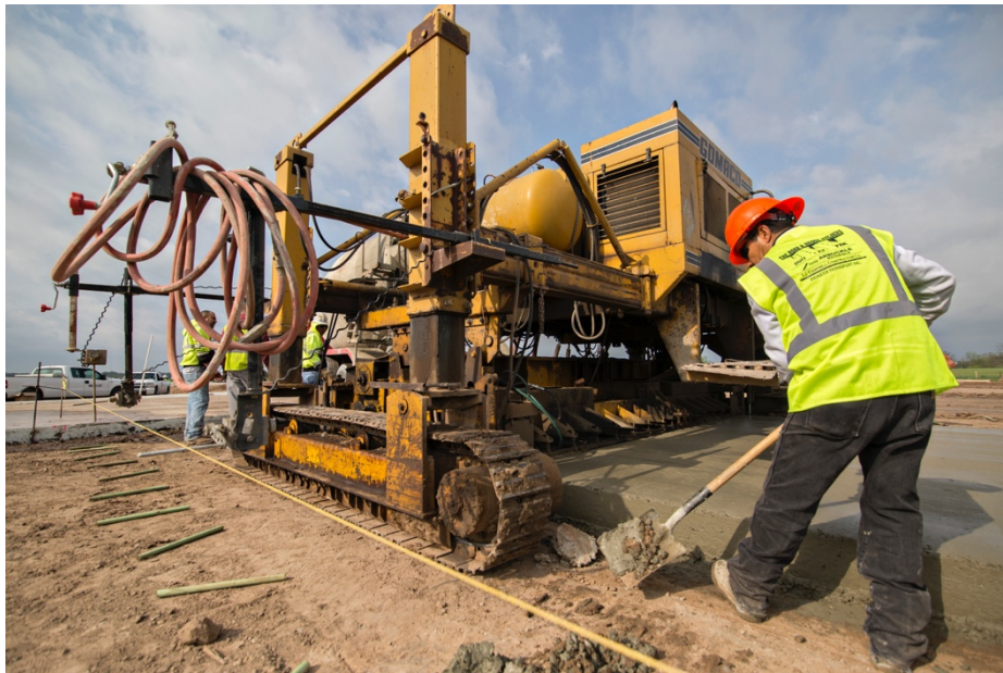
Construction of the Citizen Potawatomi Nation Iron Horse Industrial Park and Foreign Trade Zone near Shawnee, OK. When complete, this 400-acre park will provide access to rail and road networks for industrial and manufacturing tenants.
